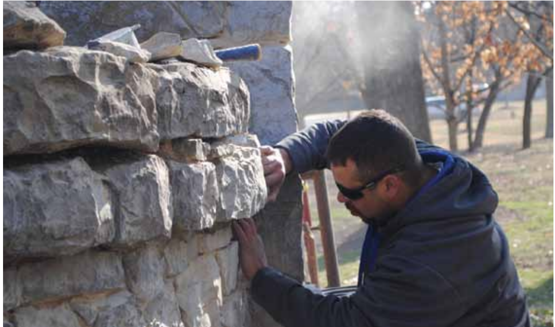
A workman from WASCO places new stone into the side of the Arch to replace rock that has been broken and chipped away as a result of the structure's exposure to the elements.
